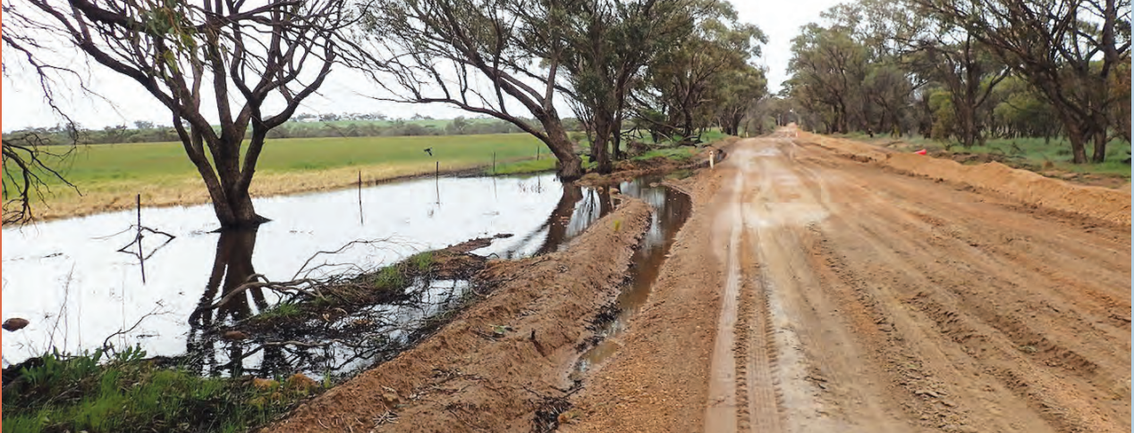
Wet conditions on the verge of along Youraling Rd will result in expensive trail construction.
